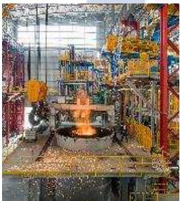
50t VD-VOD plant with mechanical pumps FRISA, Mexico
