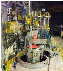
70t VD plant with mechanical pumps BOUS, Germany
