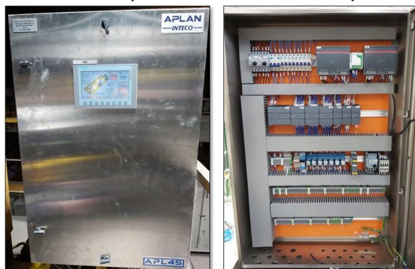
Figure 12. APL45: Main panel (PLC panel).
