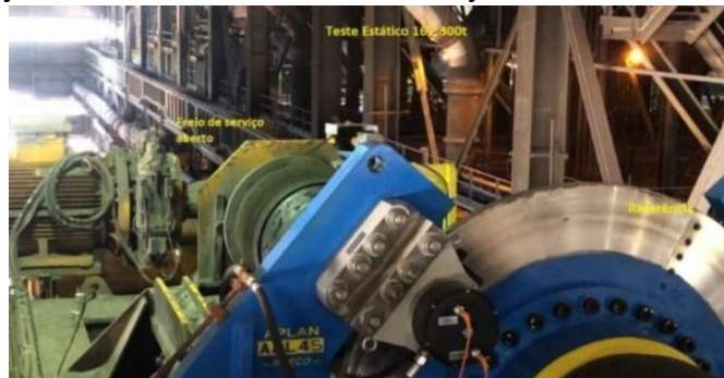
Figure 19. Service brake off.
