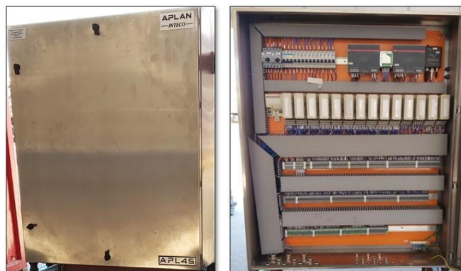
Figure 13. Remote panel and interface (crane → ABB 800xA refinery control system) Slave RF modules.
