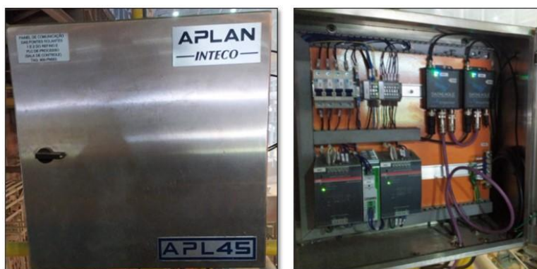
Figure 14. Interface panel (crane → ABB 800xA refinery control system) Master RF modules.
