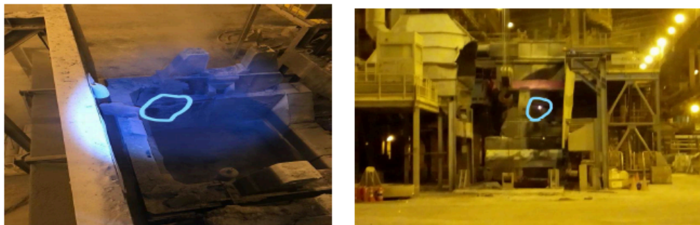
Figure 15. Example of ladle breakout and equipment damage.
